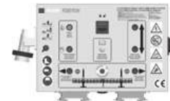
Panel with validating control system
